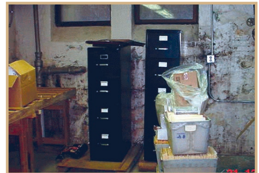
Basement prior to mold abatement.
