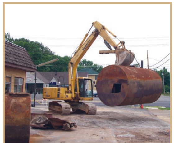
Chase licensed UST personnel comply with procedures described in the American Petroleum Institute's Publication 1604 to accomplish tank removal activities.
